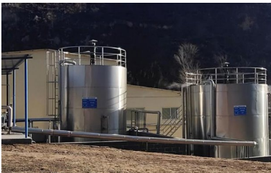
Ammonium nitrate solution storage tank
